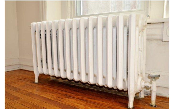
Turn on the radiator
